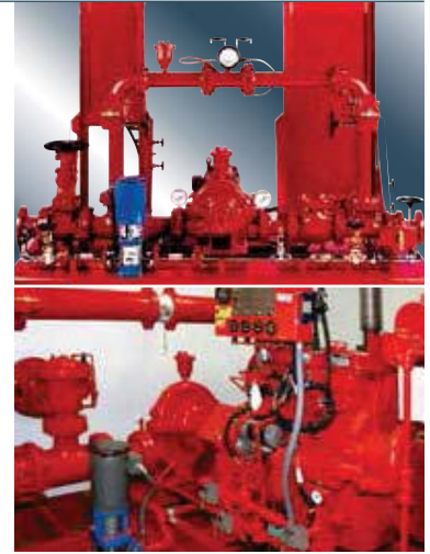
Pictured at top: Packaged Fire Pump System.
